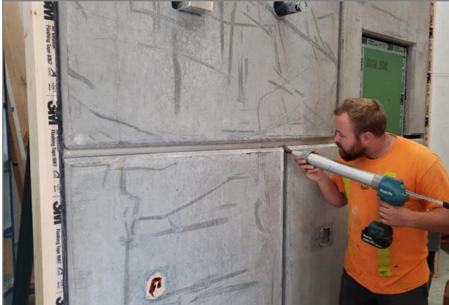
Figure 2.5 - Mock-up Wall 4, viewed from the outdoor side. Here a Stubbe's staff person is seen installing the outer seal on the 2-stage joint between the concrete panels.
