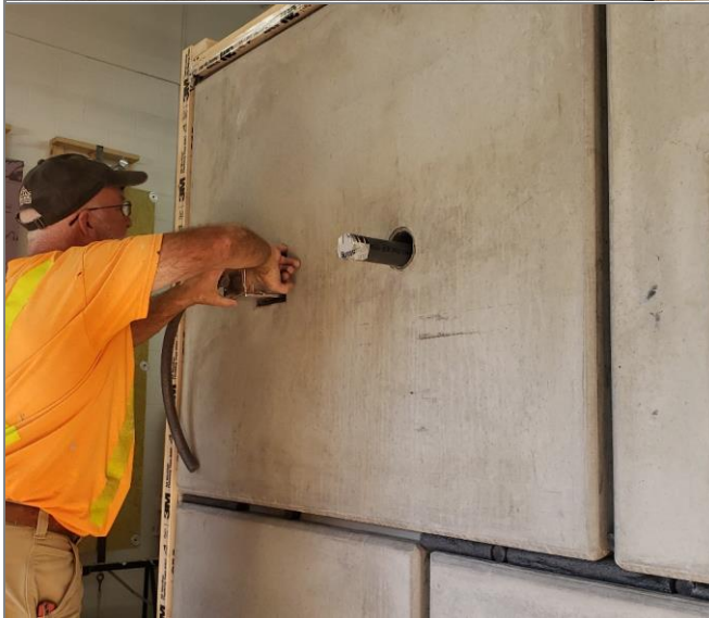
Figure 2.3 - Mock-up Wall 2, viewed from the outdoor side, showing top left concrete panel and the perimeter frame. Here one of Stubbe's staff is installing backer rod in the void between the concrete panel and the penetrating metal duct.
